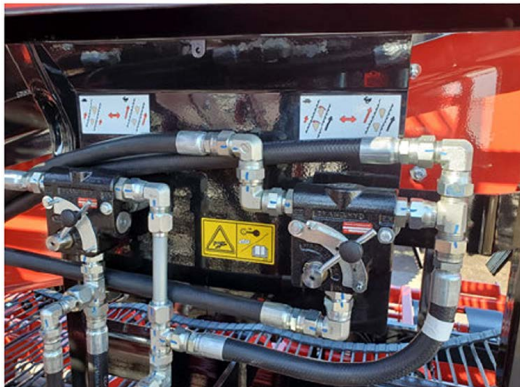
Figure 7-39: Scrub Chain Flow Control Valves
